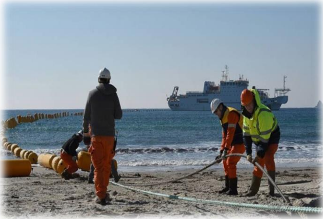
Submarine Cable Project
